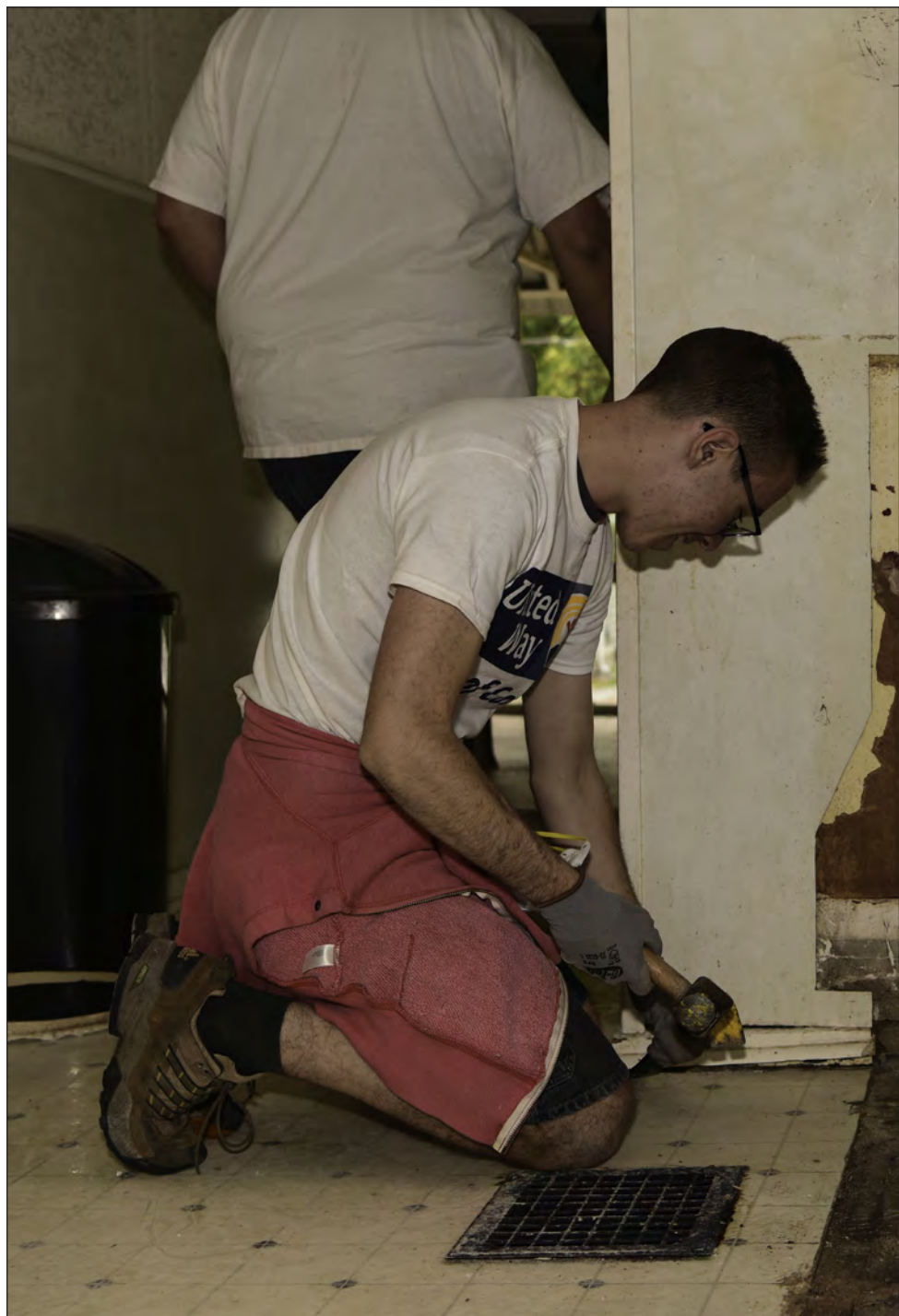
Airman 1st Class Haydn Smith, a crew chief with the 509th Aircraft Maintenance Squadron at Whiteman Air Force Base, Missouri, removes trim from a wall on Sept. 29, 2018 in Sedalia, Missouri. Smith volunteered to renovate a house that will become a shelter for homeless youth. (U.S. Air Force Photo by Airman Parker J. McCauley)
