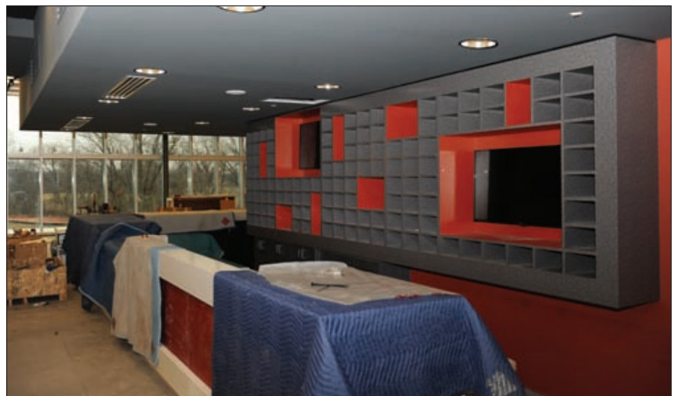
The shoe rental rack sits behind the customer service desk at the new Whiteman Bowling Center at Whiteman Air Force Base, Mo., Feb. 23, 2016. The 509th Force Support Squadron and the 509th Civil Engineer Squadron initiated the Non-Appropriated Funds Bowling Center’s construction project in 2009.
