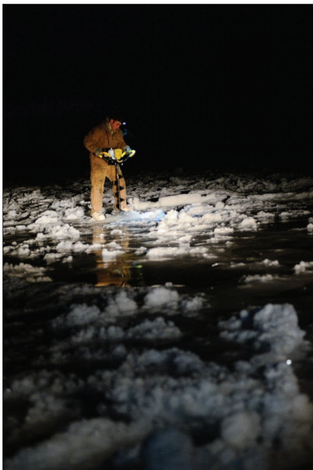
Senior Airman Tyler Dray uses an ice auger while constructing an ice bridge in Fairbanks, Alaska, Nov. 20, 2014.
