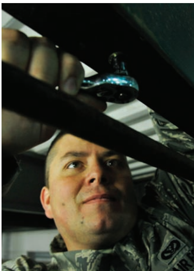
U.S. Air Force Staff Sgt. Cameron Kessinger, 509th Civil Engineer Squadron electrical systems supervisor, secures equipment to existing structure at Whiteman Air Force Base, Mo., Nov. 24, 2014. After the pipe is mounted, it must be tightened and secured to remain in place. (U.S. Air Force photo by Airman 1st Class Keenan Berry/Released)
