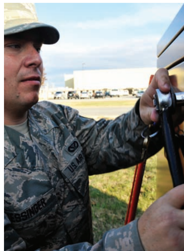
U.S. Air Force Staff Sgt. Cameron Kessinger, 509th Civil Engineer Squadron electrical systems supervisor, opens a high voltage switch at Whiteman Air Force Base, Mo., Nov. 24, 2014. This process is done to verify if the switch's configuration is in an opened or closed position. (U.S. Air Force photo by Airman 1st Class Keenan Berry/Released)
