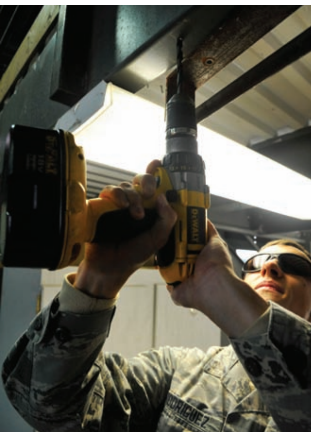
U.S. Air Force Airman 1st Class Robert Rodriguez, 509th Civil Engineer Squadron electrical systems apprentice, mounts pipe to existing structure at Whiteman Air Force Base, Mo., Nov. 24, 2014. This procedure is done to create a securing point for the pipe. (U.S. Air Force photo by Airman 1st Class Keenan Berry/Released)
